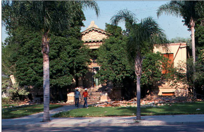
The demolition of Corona's Carnegie Library is seen here in April 1978. The site has remained an empty field ever since. Photo is courtesy of the Corona Public Library.
