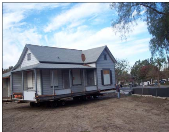
The Brumbaugh House prepped for moving, moved off its foundation, jacked up and supported by I beams on wooden cribbing.
