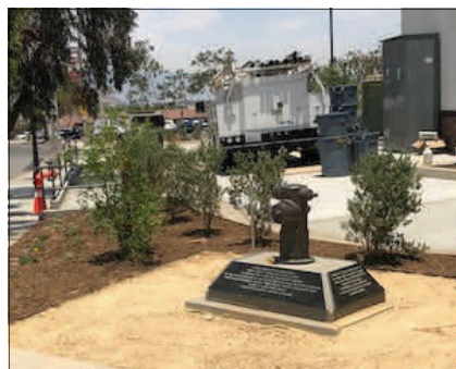
Above is an in-progress view of the existing historic marker. Main Street is at the left.
