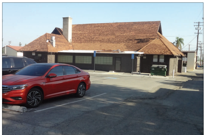
Southern exposure of completed main east-west clubhouse gabled roof, southeast corner hipped roof sunroom roof and hipped roof over kitchen.
