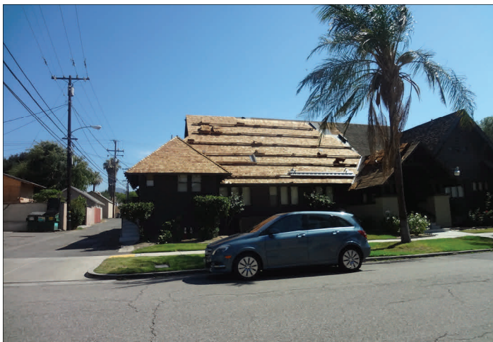
Gabled main roof north side, work in progress, old shingles remain visible on the west end, north portico roof, etc. Northeast corner hip roof has been completed, and east end of clubhouse.
