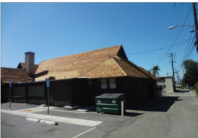
Work in progress, east end of clubhouse seen from the south, southeast hip roof, south side of gabled main roof.
