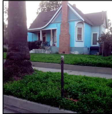
Steel tubular post with a loose steel ring at the top is located at 806 Joy Street.
